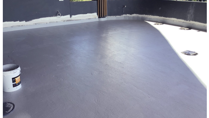
Pic 4. Apply a membrane over the screed layer - allow time to cure!
