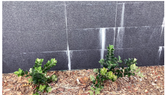
Pic 2. Porous grouts provide entry and exit points for moisture.
