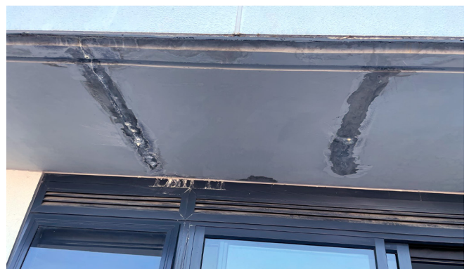
Pic 3. Left unchecked, efflorescence will weaken structures.
