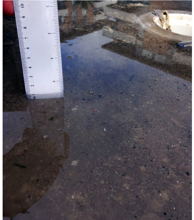
Pic 1. Incorrect drainage falls leads to ponding (refer to pic 1 & 2)
