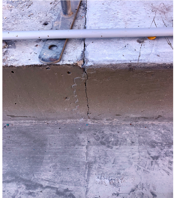
Pic 1. Flexi Bandage under membrane could've prevented cracks
