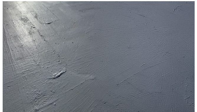
Pic 2. Uneven, irregular layers (Refer to Pic 2 & 3)
