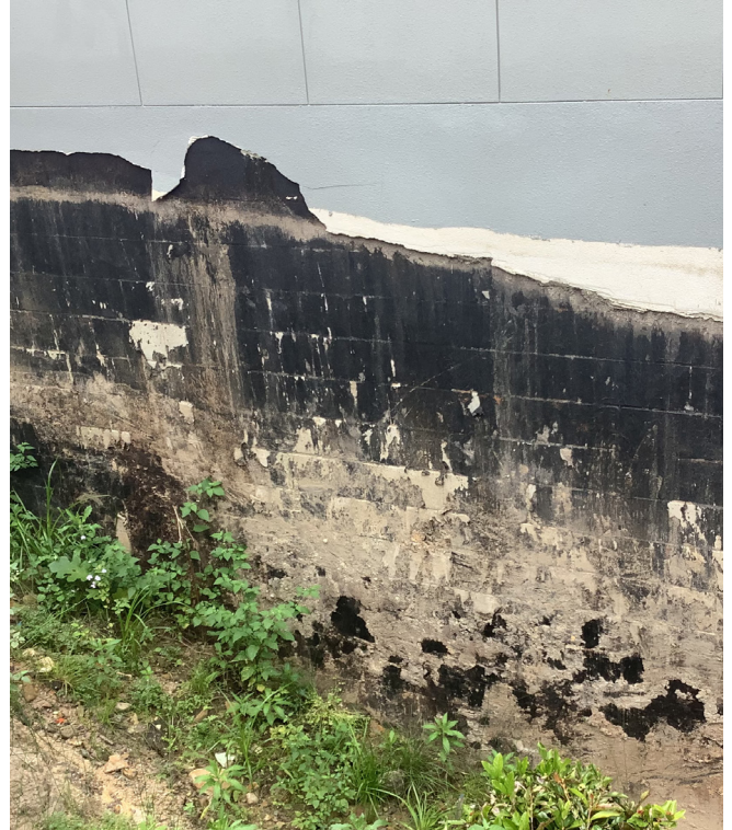
Pic 1. Failed bitumen membrane from poor prep and no root barrier
