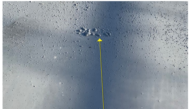
Pic 2. Outgassing caused by air pockets in porous substrates
