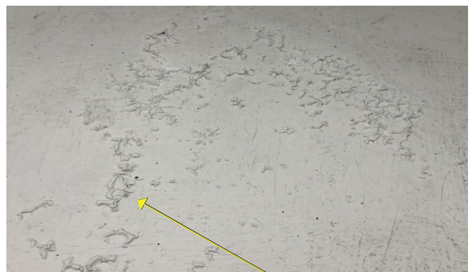
Pic 3. Bond failure at the substrate from debonding in the form of blisters
