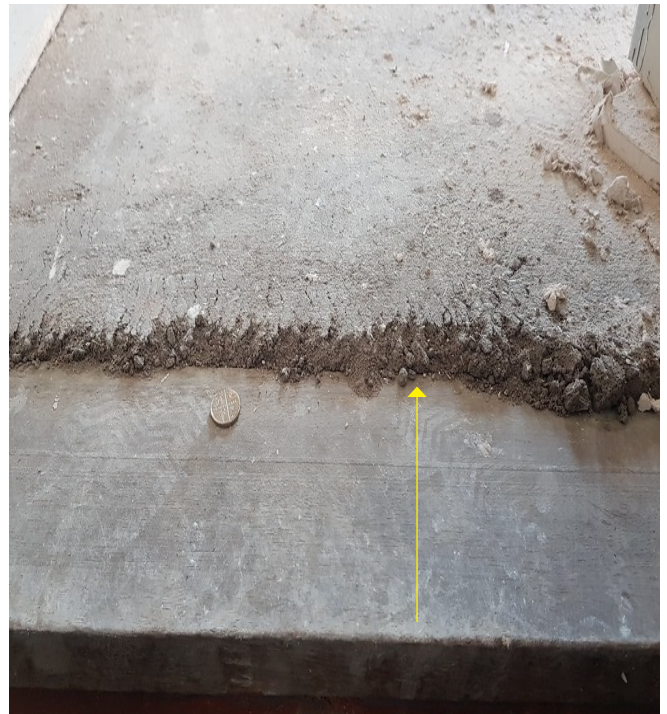
Pic 1. Crumbly Screed, incorrect MPa. Refer to Pic 1 and 2
